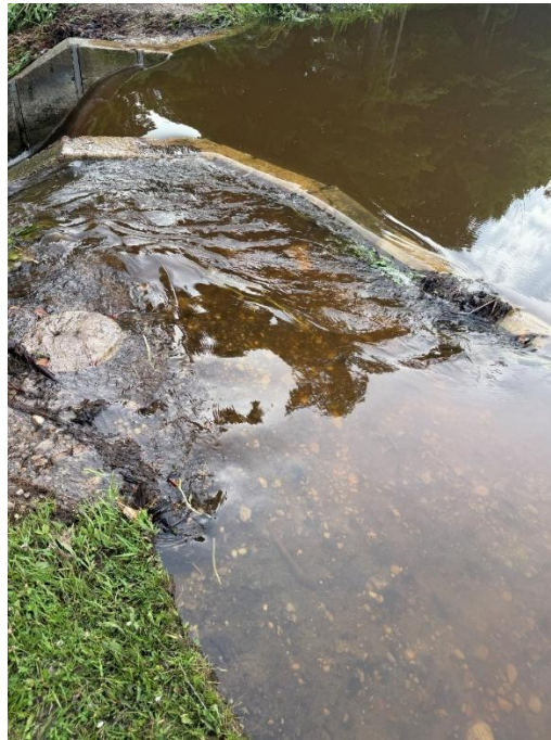
Photo 3 – Left embankment looking from the right embankment during flood as the water recedes. (6/30/2026– Provided by the Village)
