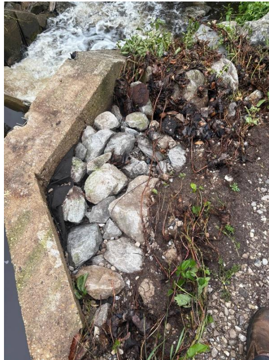
Photo 6 – Right downstream embankment along the right downstream training wall. (7/1/2026– Provided by the Village)
