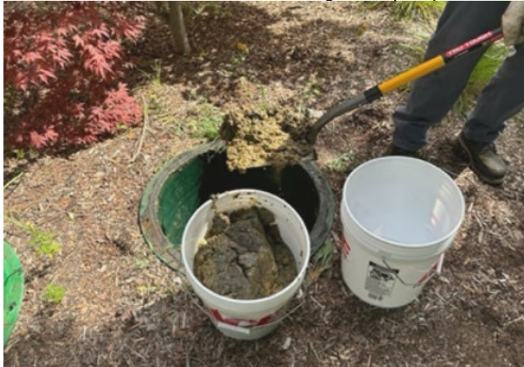
Grease removed from 110 Park St. grinder pump well
