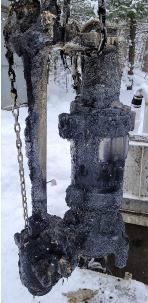
Northport Point Rd. Lift Station Pump
